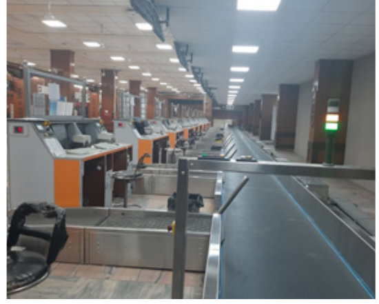
त्रिभुवामा In line baggage screening system
